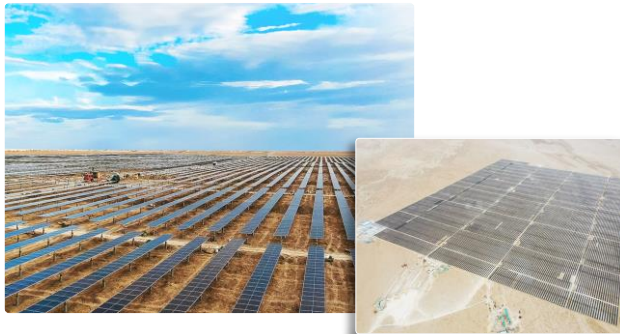
112MW On-grid Qinghai Dachaidan Power Plant
