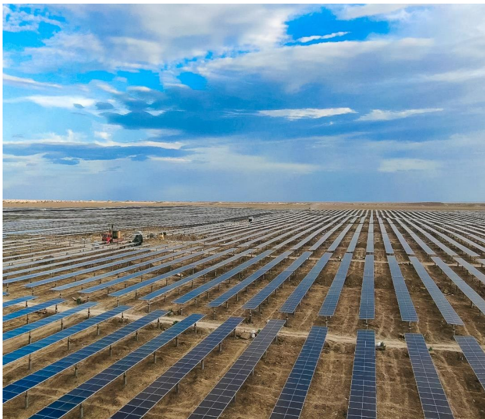
Dachaidan, Haixi, Qinghai, China 112MW Large-scale PV Project
